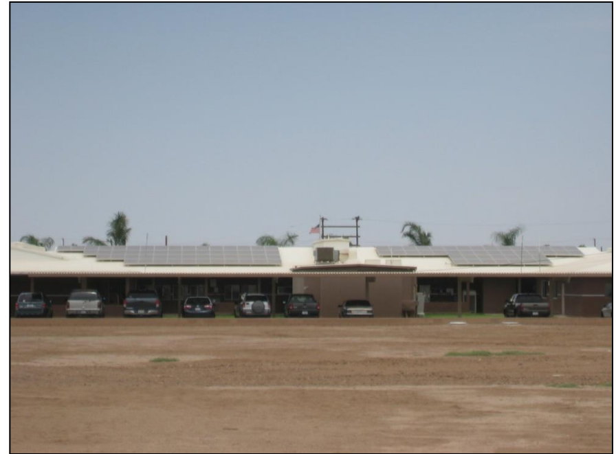
Roof Mounted Photovoltaic System
