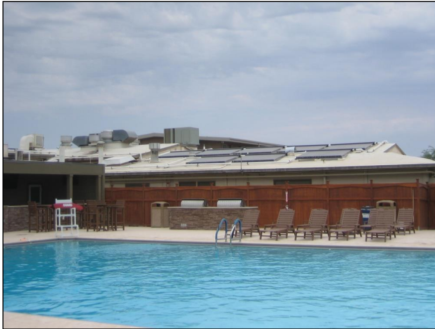
Swimming Pool Solar Thermal
